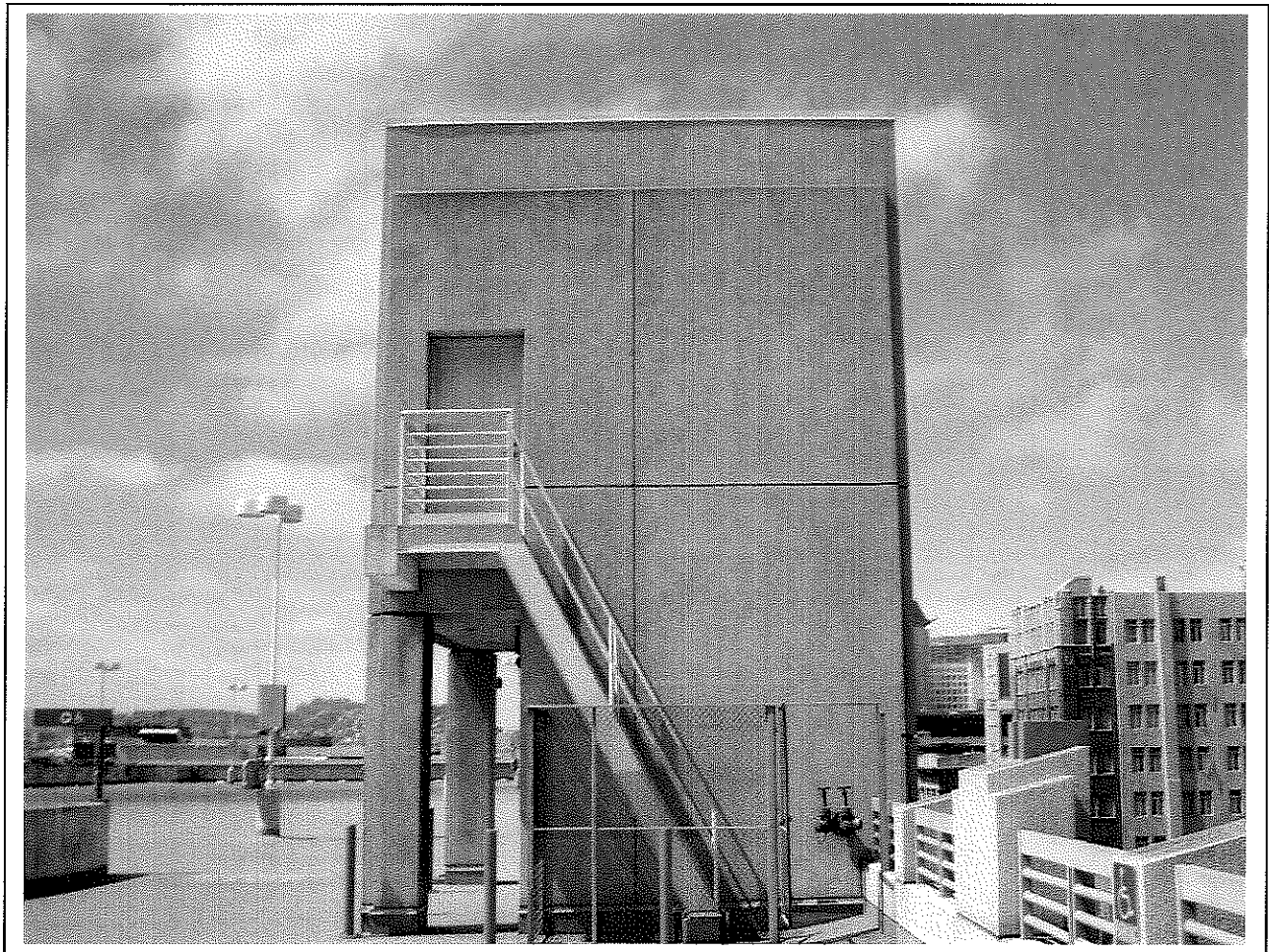
Photo of elevator/stairway structure. Proposed antenna to be placed on top via sled/ballast mount.
