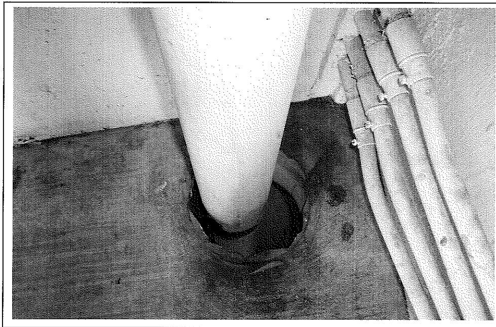
Coax cable from antenna is proposed to reach the Sprint store via core drilling down through the center stairwell. All core drilling areas will first be X-rayed to eliminate damage to structural members or other building facilities such as electrical wiring. Coax cable will be 1/2" diameter fire rated and encased in a conduit per local code.
