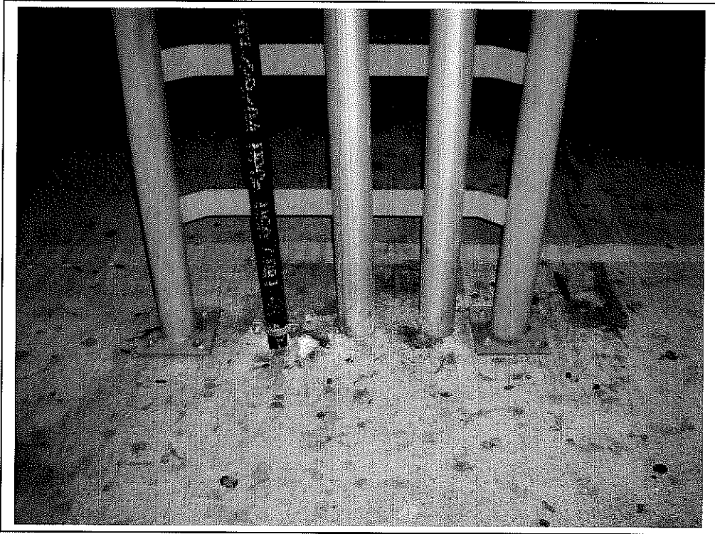
Proposed location of core drill from 2 nd level parking down into Sprint store. Note that there are existing core drills and a protective cage at this location.
