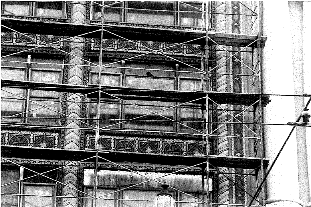
9. April 2012, Exterior Detail, North Elevation, Third Floor, Window at West, Looking S
