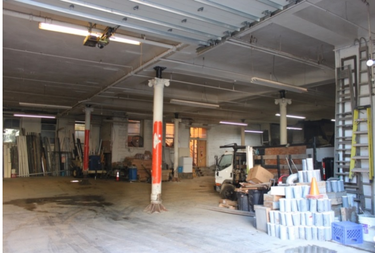
FIGURE 13. CHURCH: BASEMENT SHOWING GUTTED CONDITION, 2015.
