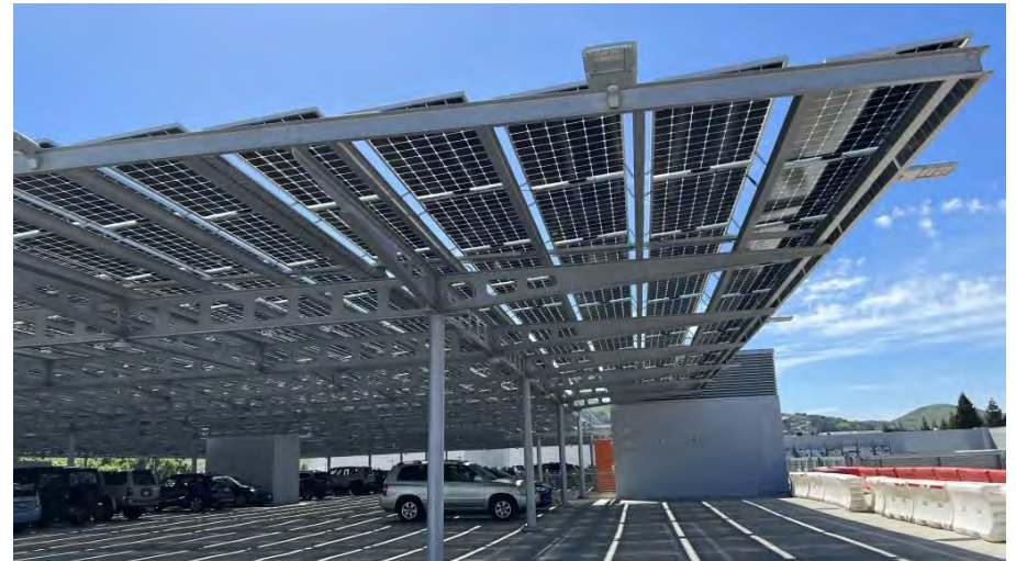
Illustrative Photo of Building with Rooftop Solar Array
