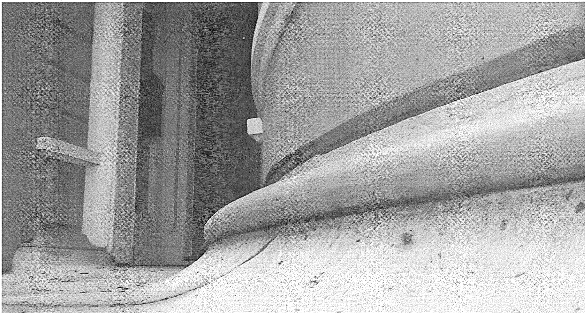
Figure 29: Detail of curb termination at wood trim (beneath area of soft deteriorated wood).
