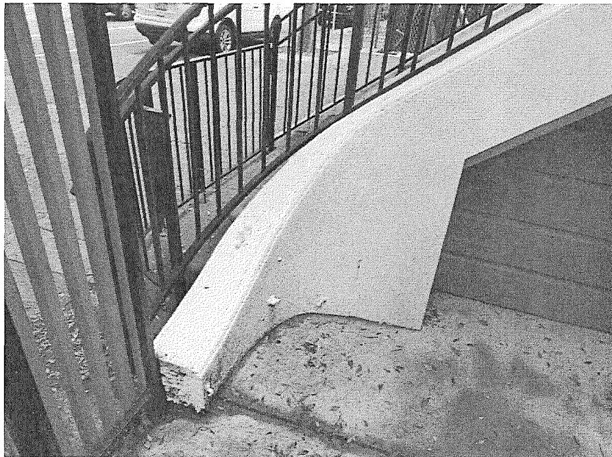
Figure 25: Detail of concrete stair curb with spall.
