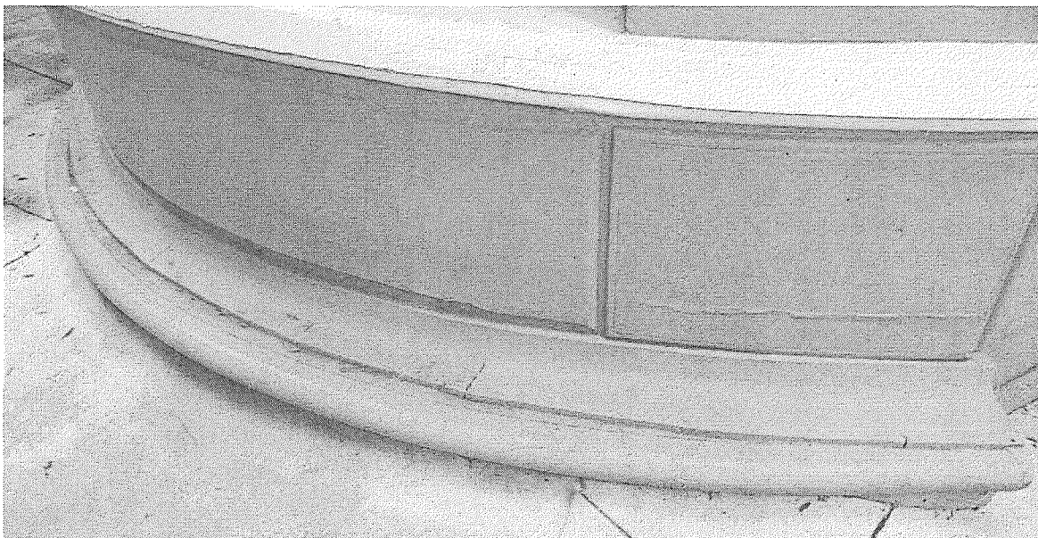
Figure 27: Detail of split wood at rusticated "block" panel and several splits at curved base trim.
