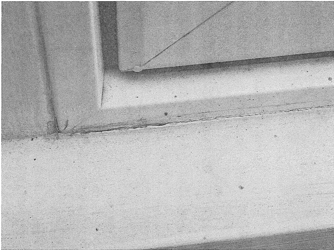
Figure 35: Detail of typical torn sealant at window perimeters.
