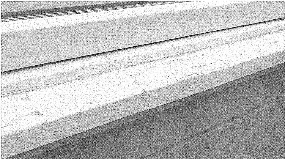
Figure 34: Detail of finger-jointed sill separation and paint degradation.
