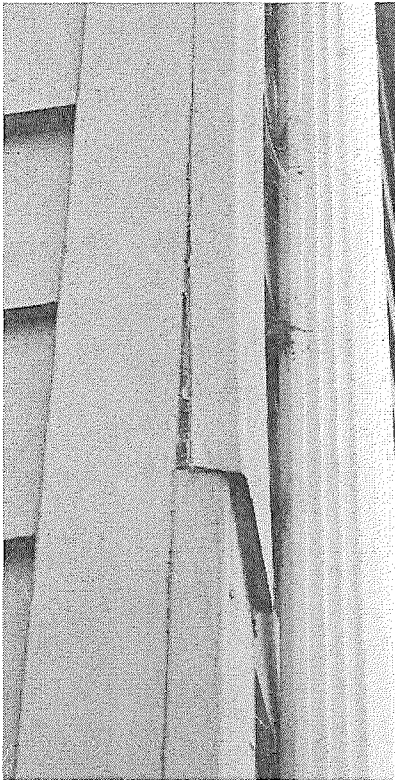
Figure 32: Example of displaced corner trim
