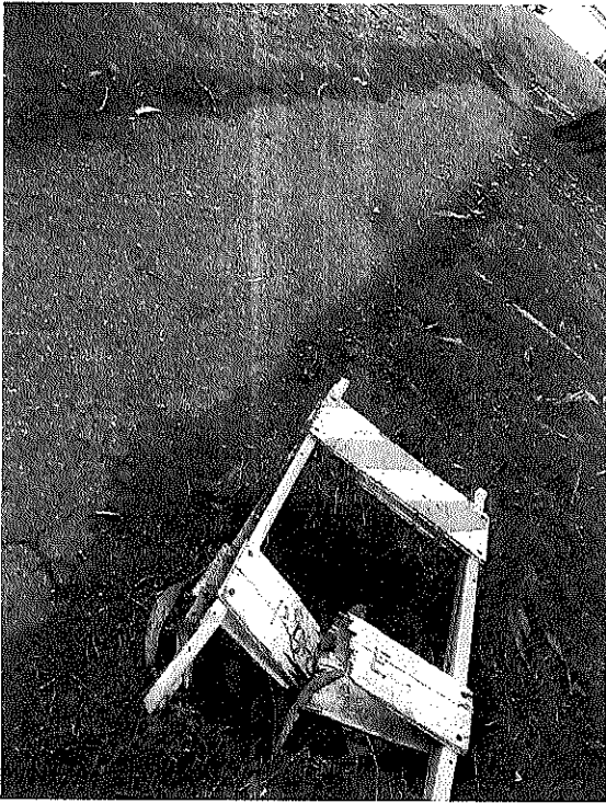
One of several abandoned holes, some two feet deep, left behind when a nearly completed plumbing project came to a halt, unfinished.
