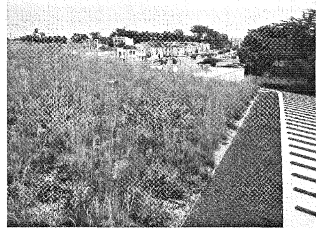
The vegetated roof at the Ortega Branch Library in San Francisco includes an Ortega Living Roof Cam that streams on their website. Photo: Robin Scheswhol
