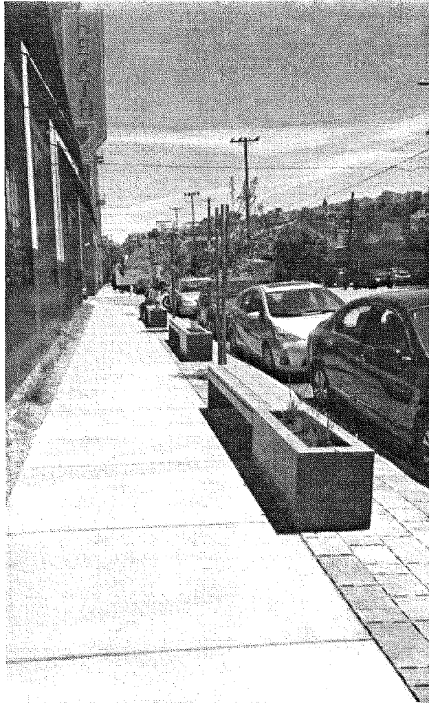
Local San Francisco manufacturer, Heath Ceramics, was awarded an Urban Watershed Stewardship Grant from the SFPUC to install permeable paving in the sidewalk along their storefront. Photo: Heath Ceramic
