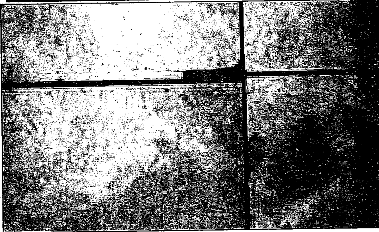
Image 16. Floor tiles unprofessional installation and damaged.
