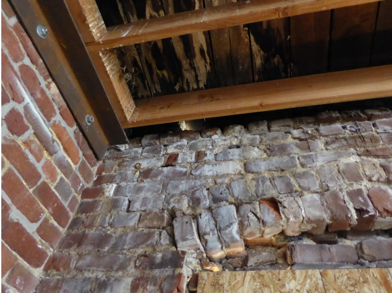
Figure 35: Detail photograph of deteriorated brick mortar joints and efflorescence above southernmost window opening at fifth level. Note rust stains surrounding metal embedments and water stains at underside of roof sheathing (photograph taken on 02/27/2018).
