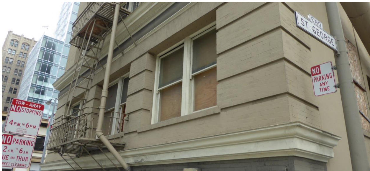
Figure 20: Detail view of brick cladding with horizontal reliefs at second floor, and typical wood double-hung windows. Note materials on the north façade (brick and water table bands) continue onto the west façade for a few feet (photograph taken on 01/26/2018).
