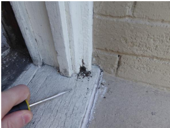
Figure 39: Detail photograph of typical deterioration at window trim (Photograph was taken on 02/27/2018).
