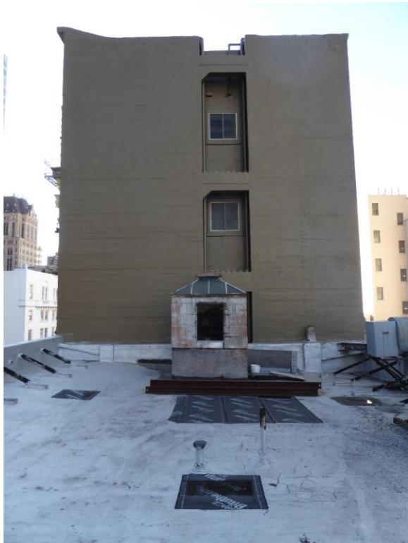
Figure 46: Photograph of roof, looking south towards elevator penthouse and adjacent building (photograph taken on 02/27/2018).
