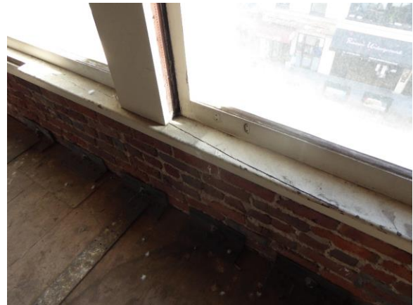
Figure 40: Detail photograph of split window sill (photograph taken on 02/27/2018)
