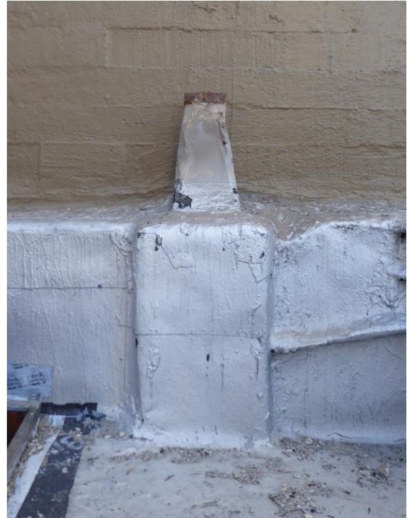
Figure 49: Detail view of open flue at southern parapet wall (photograph taken on 02/27/2018).
