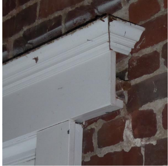
Figure 42: Detail photograph of window cornice and edge of concealed steel lintel behind (photograph taken on 02/27/2018).
