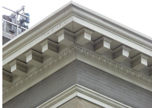
Figure 19: Detail photograph of denticulated sheet metal cornice and brick frieze. Note localized paint peeling at cornice (photograph taken on 01/26/2018).
