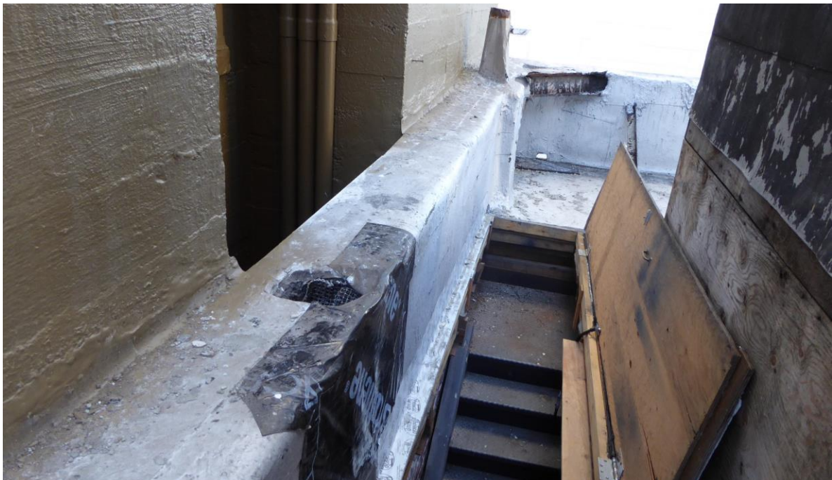
Figure 50: Photograph of roof access hatch located between elevator penthouse and southern parapet wall (photograph taken on 02/27/2018).
