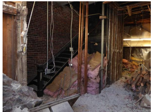
Figure 28: Interior view looking southwest towards entry bay and metal stairs to second floor. Photograph taken from second bay entry (photograph taken on 04/02/2018).
