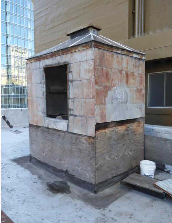
Figure 48: Photograph of elevator penthouse clad in metal panels over wood sheathing. Note surface corrosion on metal panels and missing access door (photograph taken on 02/27/2018)
