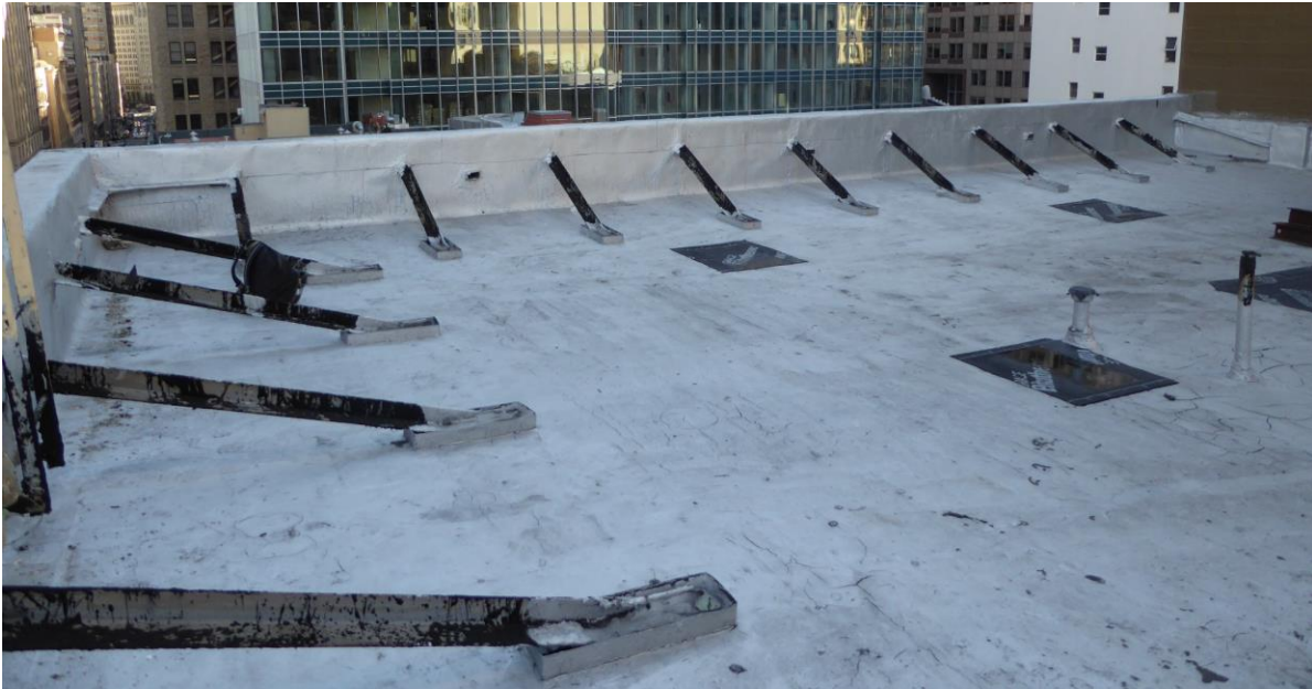
Figure 45: Photograph of built-up roof, looking east. Diagonal seismic bracing supports parapet walls (photograph taken on 02/27/2018).
