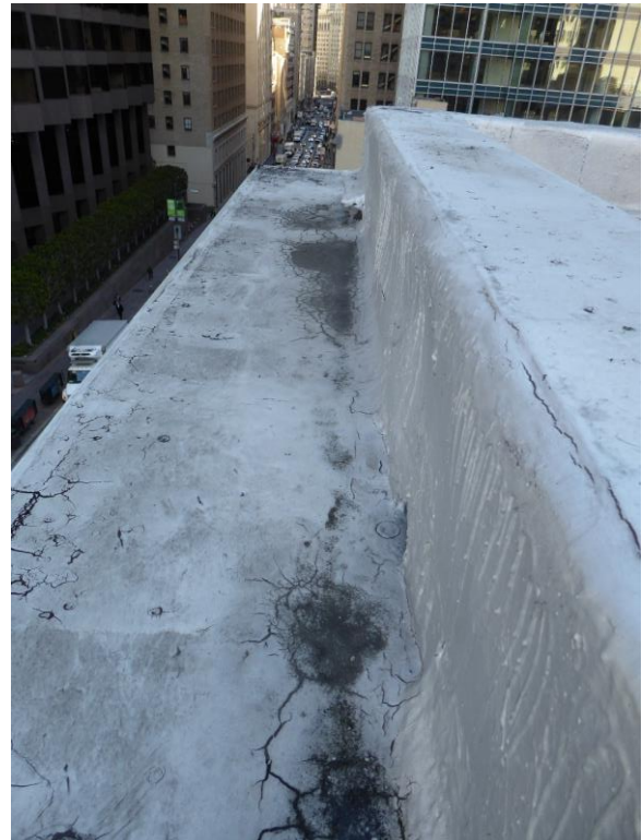
Figure 47: Detail view of parapet and top of cornice. Through-wall scuppers at the northern and eastern parapet walls drain the cornice back to the roof (photograph taken on 02/27/2018).
