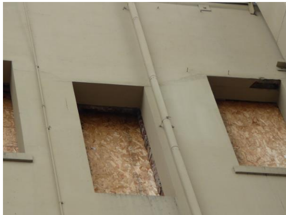
Figure 23: Detail view of punched openings. Note cracked cement plaster between window lintels (photograph taken on 01/26/2018).
