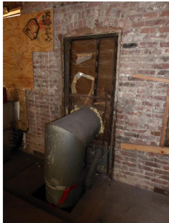
Figure 34: Detail view of punched window (original door) opening with ventilation duct. Note deteriorated wood frame (photograph taken on 02/27/2018).
