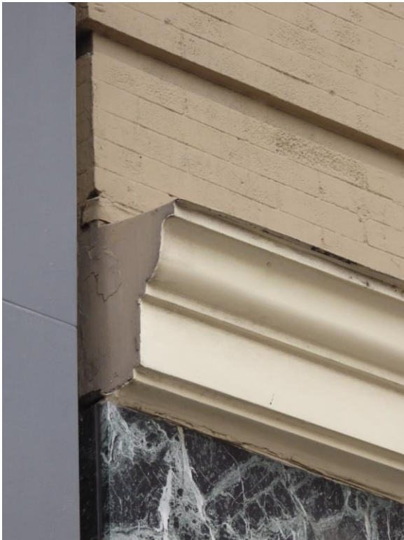
Figure 16: Detail photograph of sheet metal water table banding at second floor. Note brick erosion beneath the paint on the brick substrate (photograph taken on 01/26/2018).
