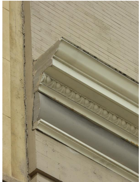
Figure 17: Detail photograph of water table banding at the third floor. Note minor spot corrosion bleeding through the paint (photograph taken on 01/26/2018).
