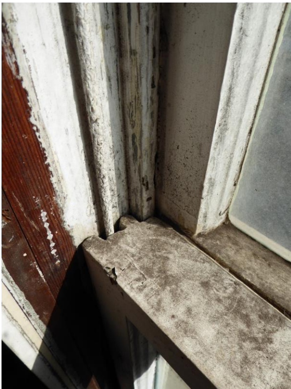
Figure 43: Detail photograph of top edge of lower sash, and sash cord. Note typical paint chipping and missing sash stop (photograph taken on 02/27/2018).
