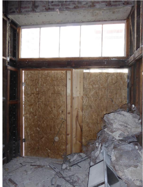
Figure 26: Interior view of storefront at second bay along Kearny Street. Note historic wood and glass transom above infilled plywood (photograph taken on 04/02/2018).
