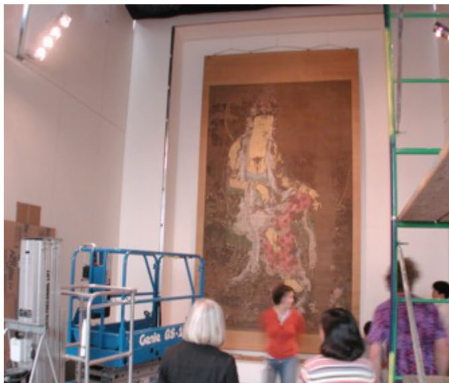
Kagami Jinjya Exhibition Installation - A new interior wall and display case was built over the glass curtain wall of the North Atrium to display this exhibit.
