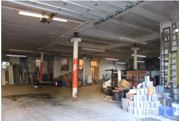
FIGURE 13. CHURCH: BASEMENT SHOWING GUTTED CONDITION, 2015.
