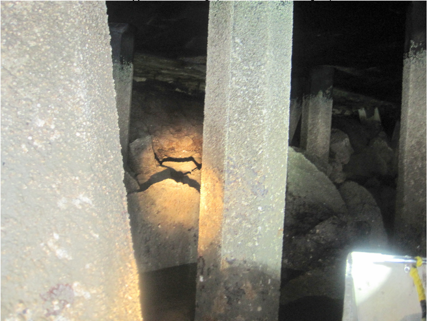
Photo 5. Undermining of seawall
