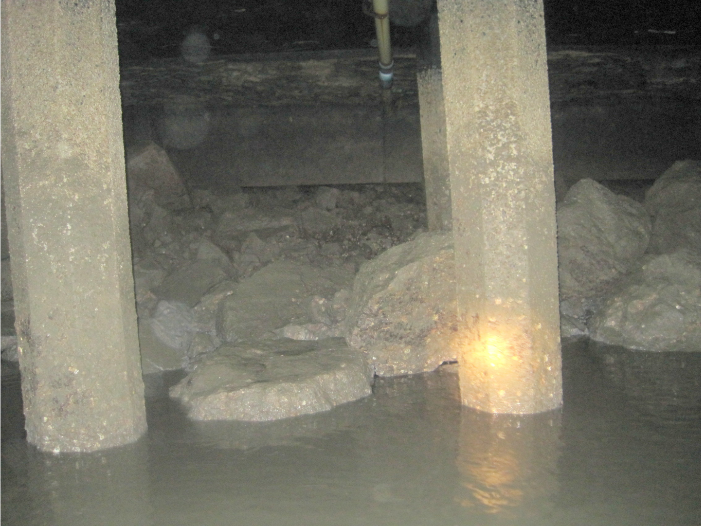
Photo 1. Undermining of rip-rap and slurry may be present
