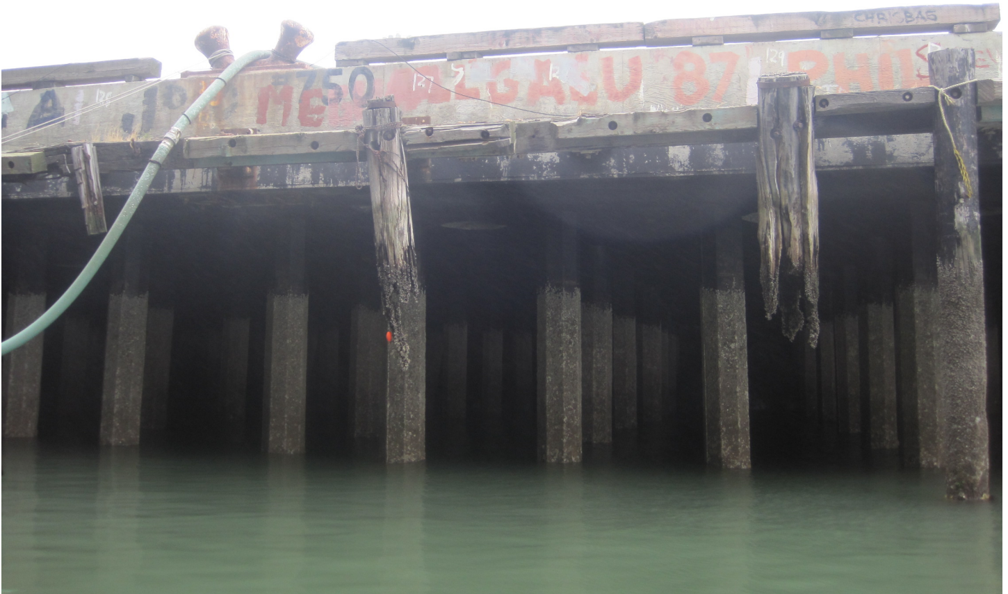
Photo 6. Hanging wood members
