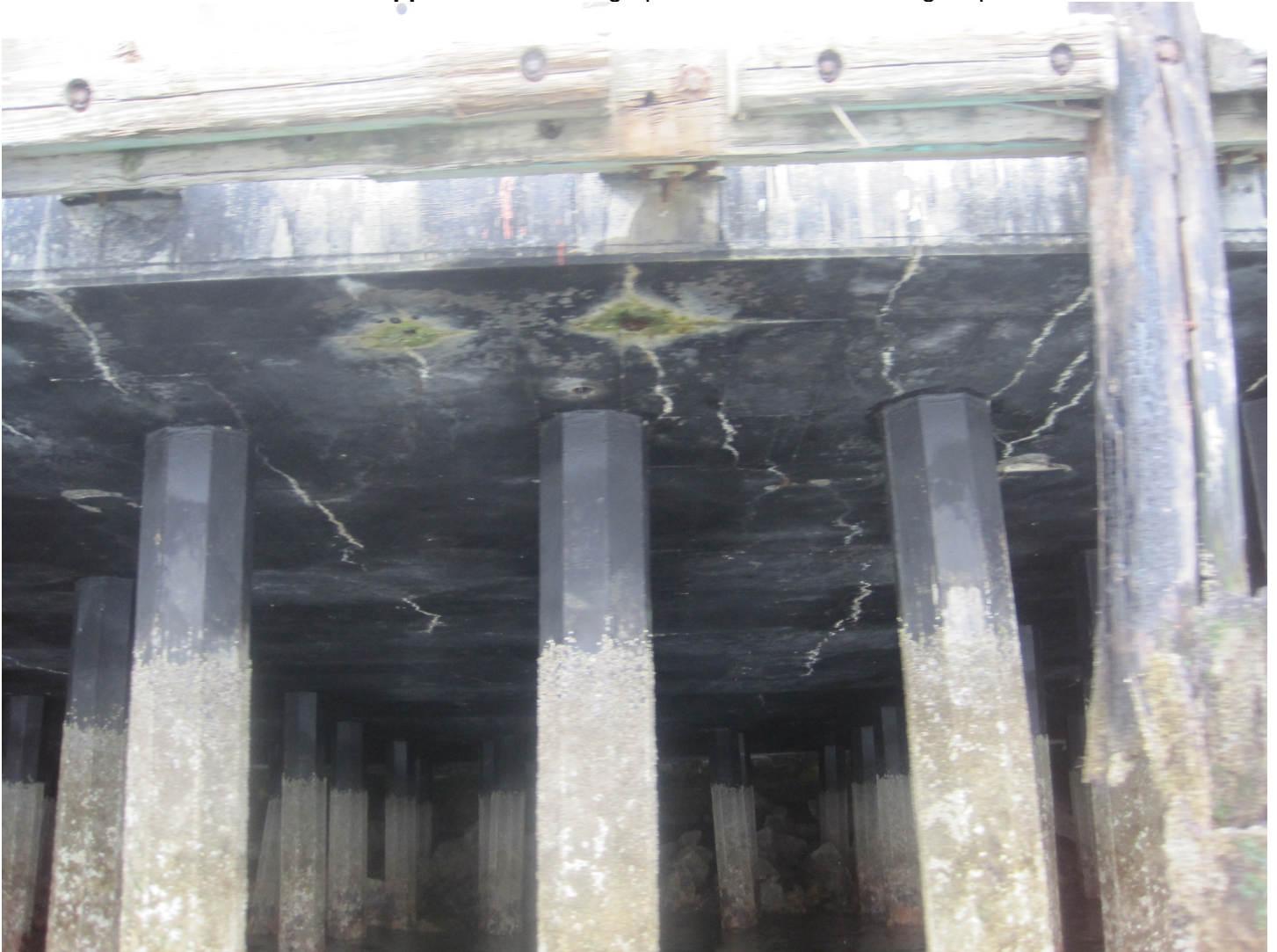
Photo 4. Cracks in concrete deck
