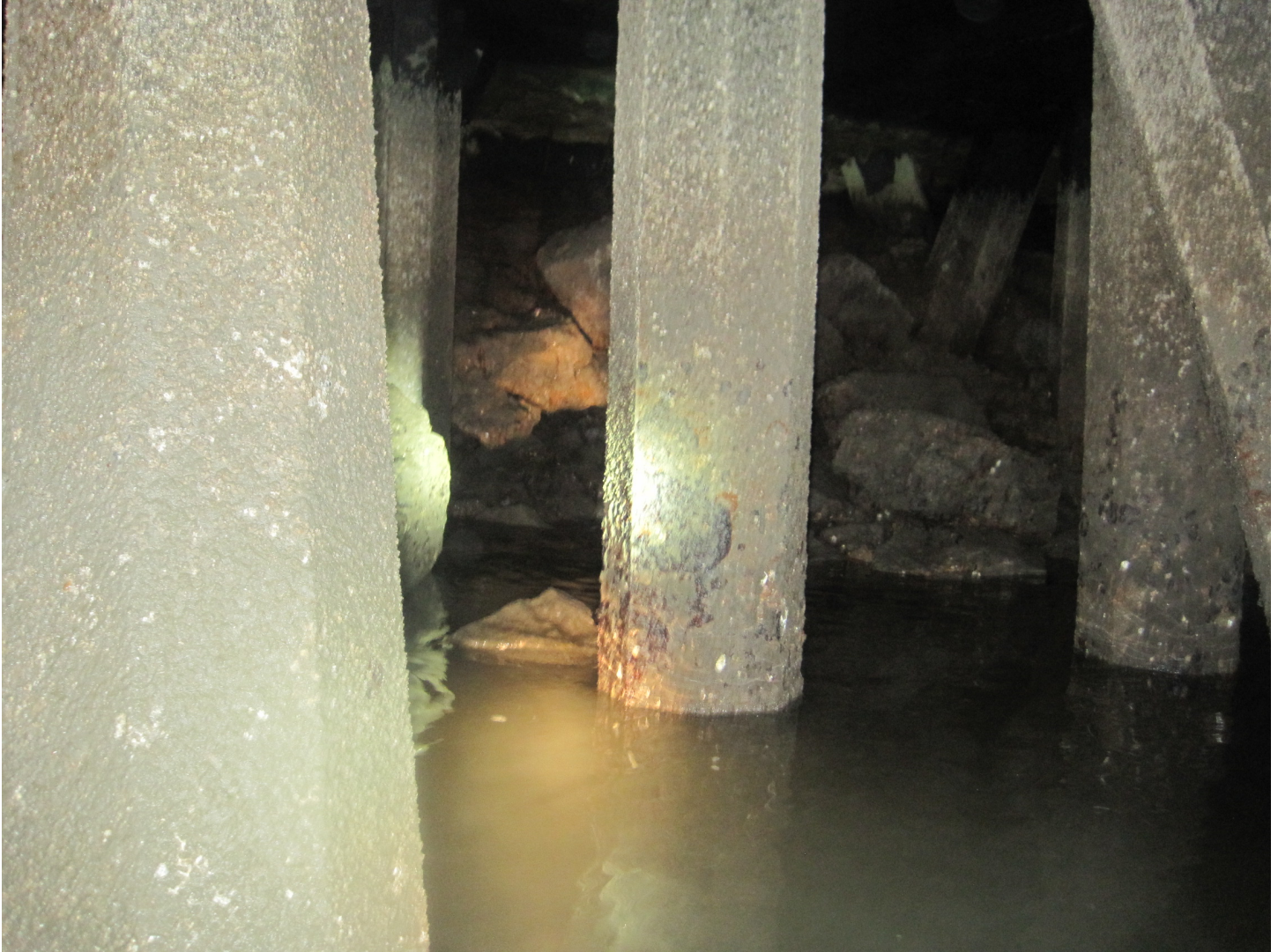
Photo 6. Undermining of seawall
