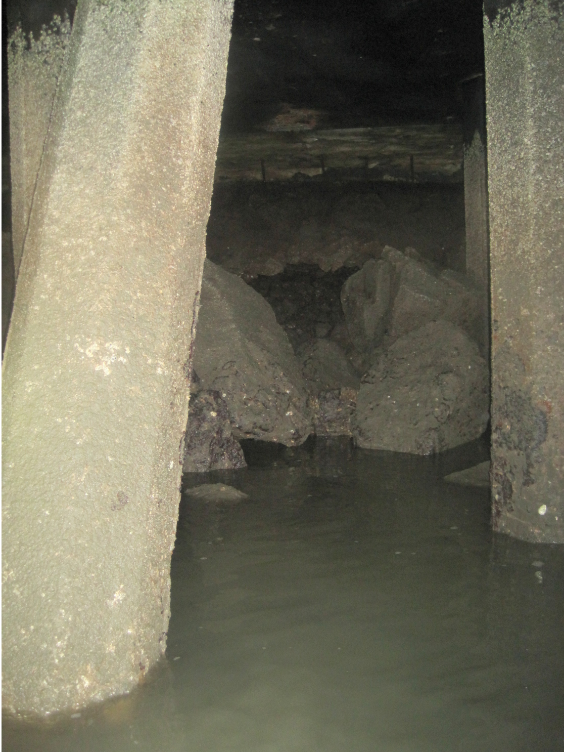
Photo 3. Undermining of seawall
