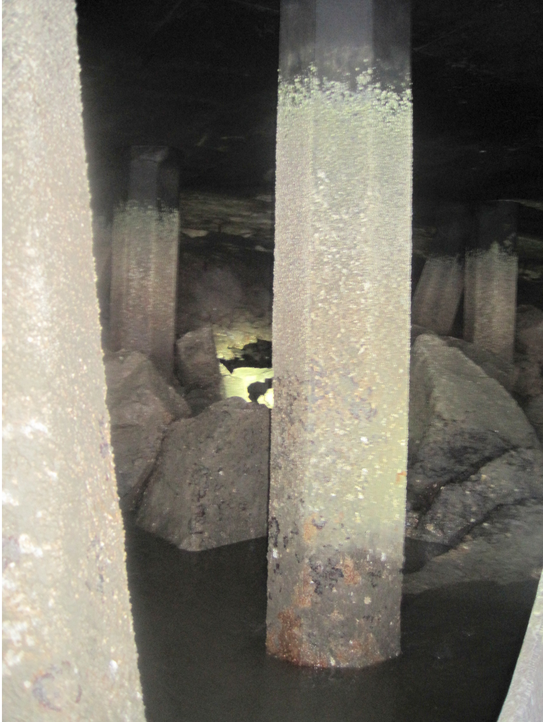
Photo 4. Undermining of seawall
