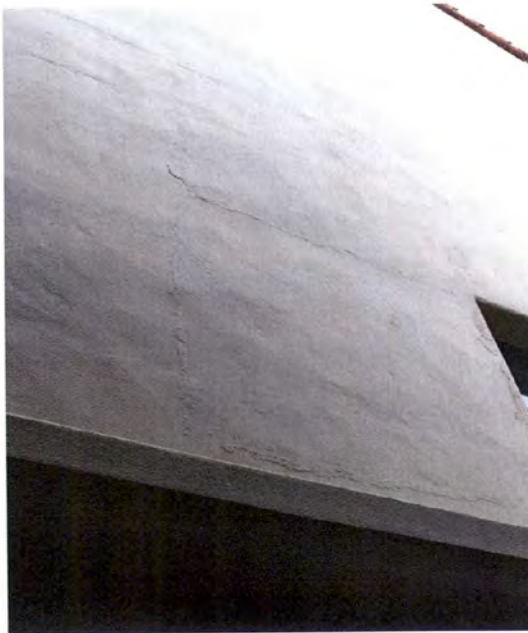
Figure 22 - Visible bulging at the crack repair on the east facade of the Annex; there is the potential here for failure in the future. Photo by Page & Turnbull
