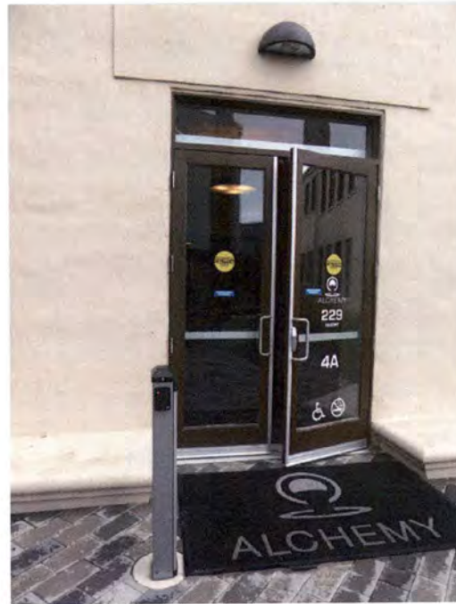
Figure 13 - The ADA pushplates at these courtyard doors only open the door this much. Photo by Page & Turnbull, 2017.
