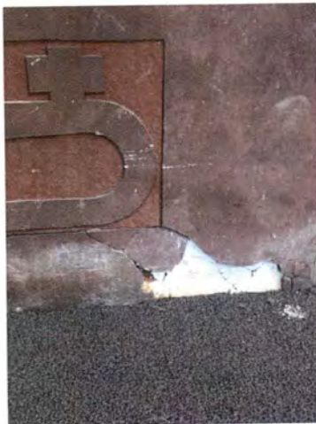
Figure 30 - Spalling and cracks at the mural base
