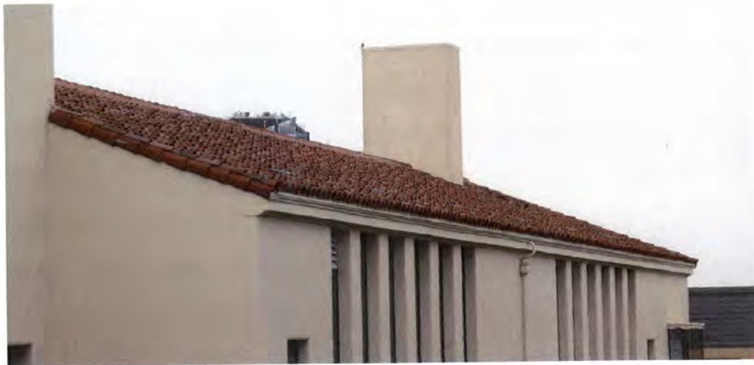
Figure 24 - The roof on Woods Hall Annex in good condition. Photo by Page & Turnbull
