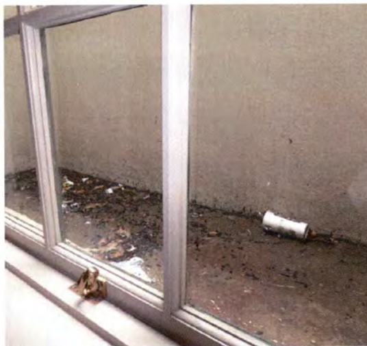
Figure 17 - Debris and trash in the lightwell. Photo by Page & Turnbull, 2017
