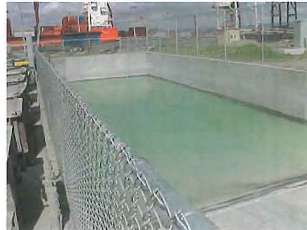
Rainwater harvesting is a volume-based BMP that can be used to collect water for various types of industrial operations, resulting in reduced utility costs.
