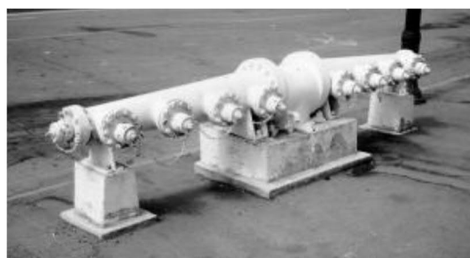
Figure 2-5: Typical Fireboat Manifold Inlet
