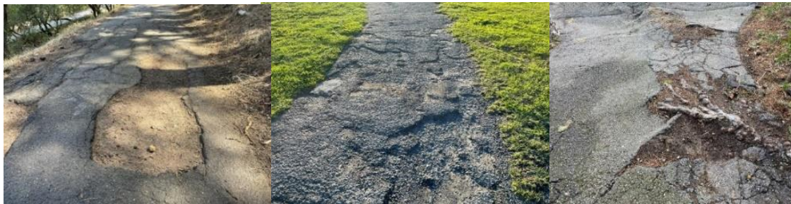
Figure 1. Defective Pathways in Buena Vista Park, Lincoln Park, and Brooks Park
