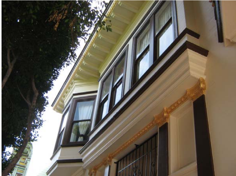
View looking southeast at upper level of primary façade. Source: Page and Turnbull
