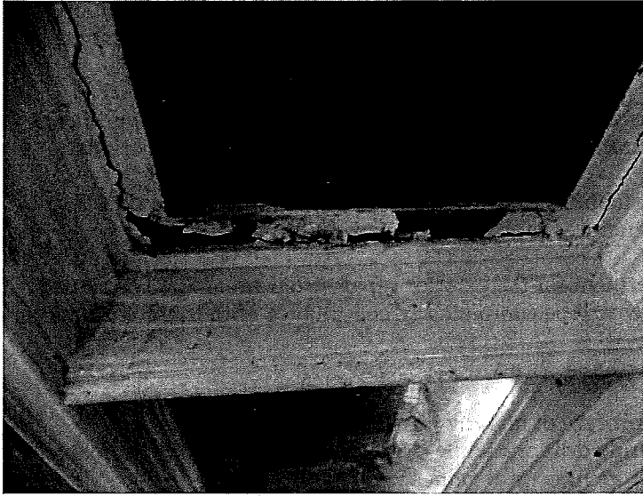
Figure 22. Peeling paint and corrosion at ground floor window. (Photograph by Garavaglia Architecture, Inc., April 2015.)
