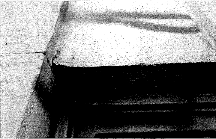
Figure 18. Cracked concrete above window at the seventh floor along the north elevation. (Photograph provided by RLJC, April 2015.)
