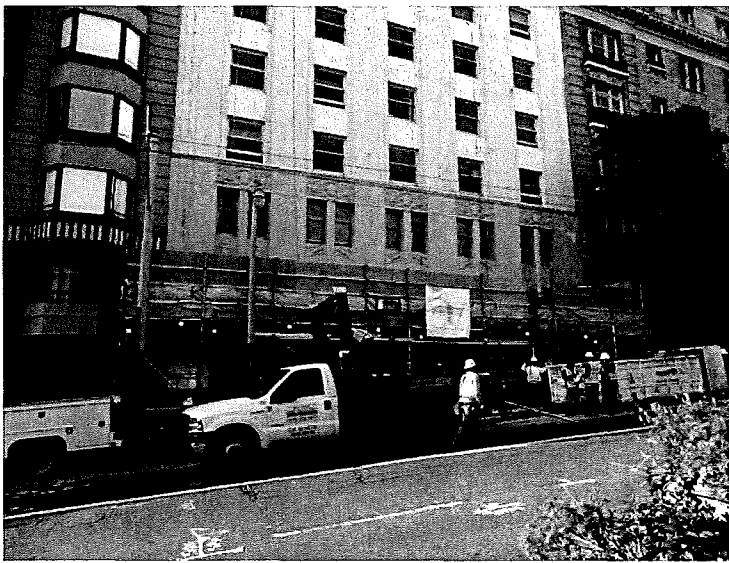
Figure 8. Overview of north (Post Street) elevation, showing first two floors of building. (Photograph by Garavaglia Architecture, Inc., April 2015.)
