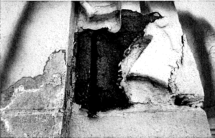
Figure 19. Exposed reinforcing bar at the twelfth floor along the north elevation. (Photograph provided by RLJC, April 2015.)
