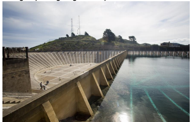
Twin Peaks Reservoir joint sealant
