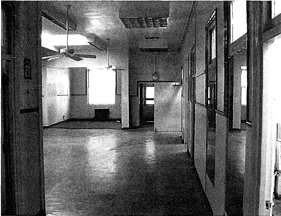
Former ward room, view northwest; note cream-colored tile with tan-colored tile borders.
