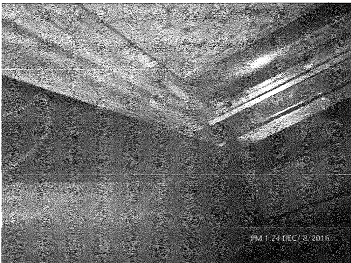
Test site ST5 in unit 31B heat pump closet. Note test smoke flowing up through heat pump closet door opening
