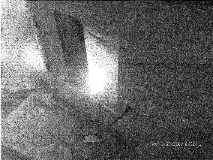
Test access opening in bedroom wall at site ST1 in unit 31B
