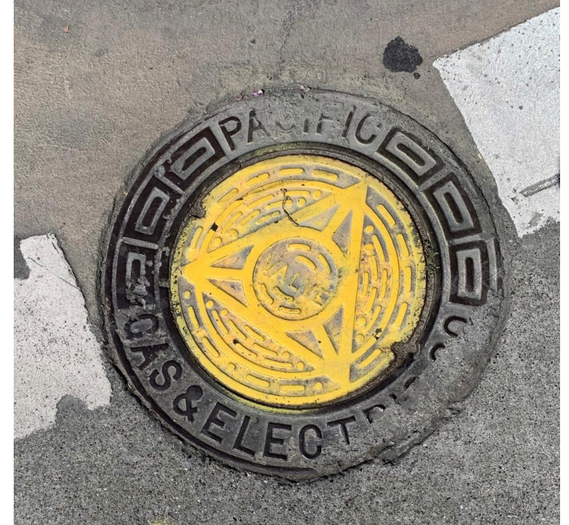
Emergency Shutdown Zone Valve identified by yellow cover
